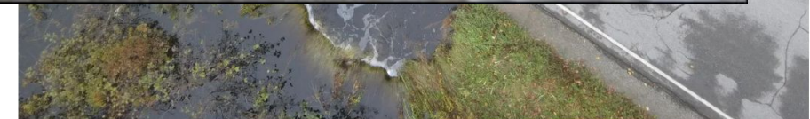
A portion of Pushaw Road in Glenburn collapsed last Saturday when heavy rain washed away one of culverts that carries a stream under the road. The Maine Department of Transportation is working to repair the damage, but it will likely take several days. Credit: Courtesy of Andy Ryder of the Glenburn Fire Department
